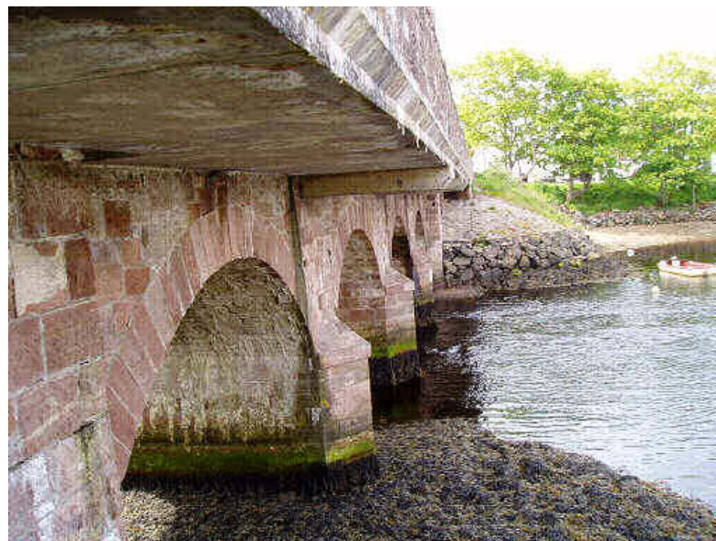
Plate 3.18 - Arch bridge at Cushendun, widened using a cantilevered structure, similar to what is proposed for the Callan River Bridge on the Killylea Road
