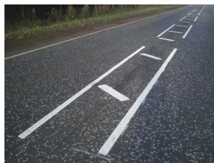
A section of the Ladder Markings
