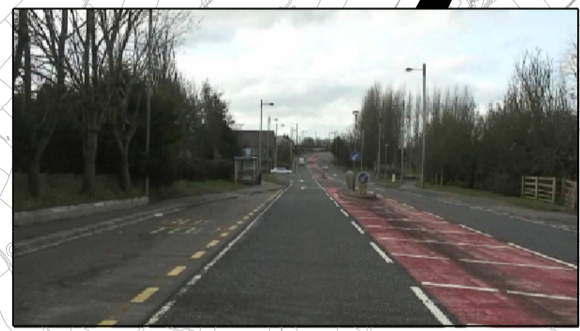
Footway of varying width and condition along the Eastern verge terminating at the Western properties of Ballynure
