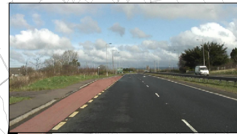
1.5m footway situated in Eastern verge, terminating at the property adjacent to Rushfield Road
